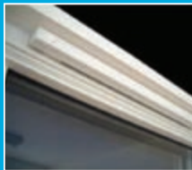
Improve air flow by leaving trickle vents open on all windows or leave windows open (if safe)
